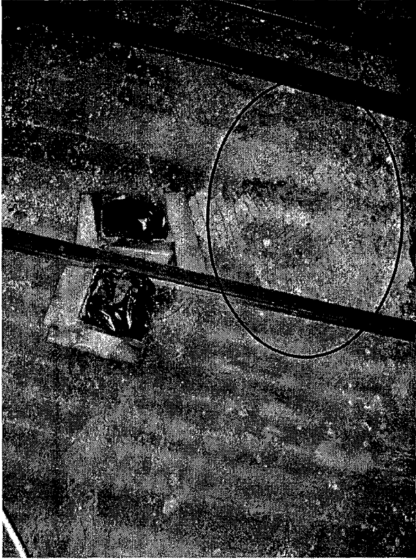
Hole in Attic Roof & Vent
